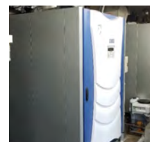
A waste cooking oil boiler
