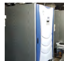
A waste cooking oil boiler
