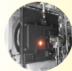
Boiler facility for incinerating chicken droppings
