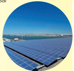
Solar panels on roof
